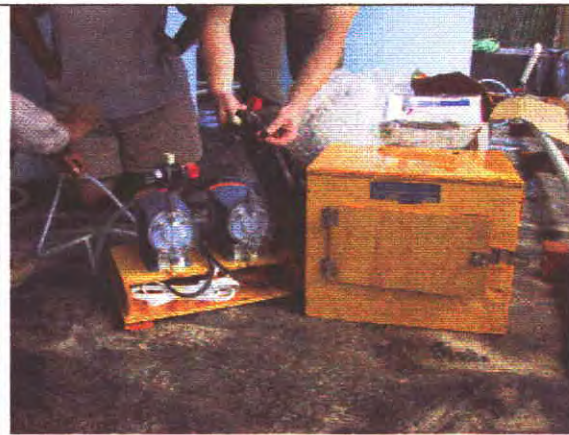
Figure 4. Assembly of diaphragm pumps and backpressure valves
