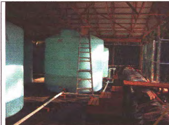
Figure 3. Storage Tanks and Protective Berm-Liner for Ammonium PolyPhosphate Nutrient
