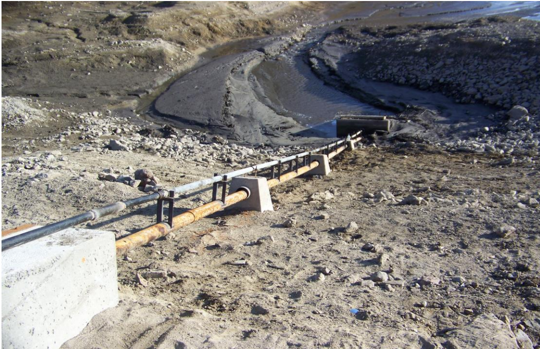
Figure 8. Looking downslope, the repaired pipe and protective tube stretch from the top of the dam to the gate box at the outlet. Newly fabricated H-brace vertical supports hold valve stem and tubing secure.
