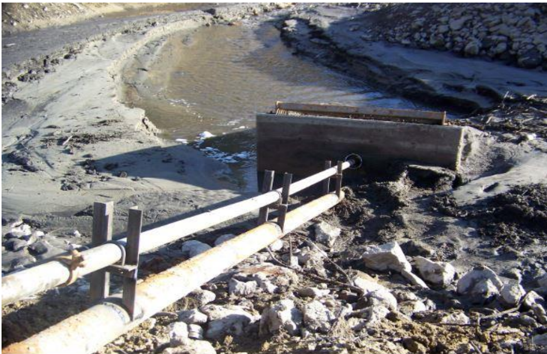
Figure 9. View of pipe and valve stem tubing entering the gate box at the outlet. The raised gate, just visible above the gate box, signifies the valve is wide open during testing of the dam structure after repairs.
