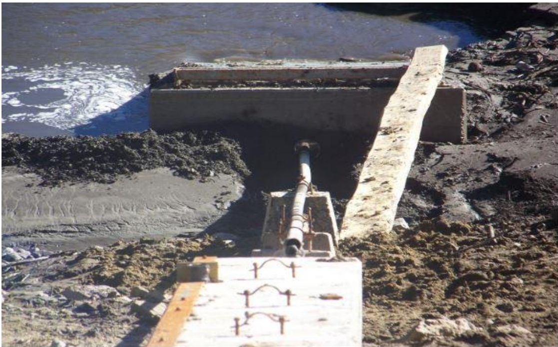
Figure 7. Closer view of damaged, bent pipe with the smaller valve stem visible inside the pipe connected to the front of the gate box. Wood plank at right was used to access the gate box.
