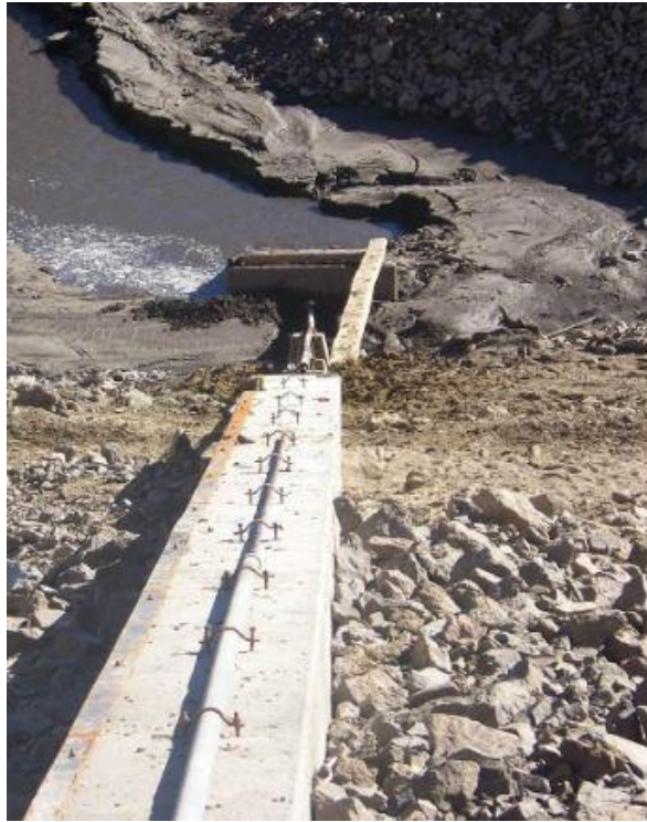
Figure 6. Repaired valve stem and protective tube leading from the top of the dam at Mosquito Flat Reservoir downhill toward the gate box at the outlet. Damaged pipe is visible in front of the gate box.
