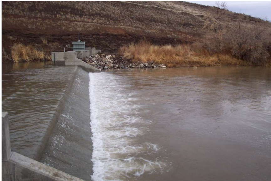
Figure 43. Pictures of the Hot Springs Diversion Dam after site dewatering (top photo) and after project completion (bottom photo).
